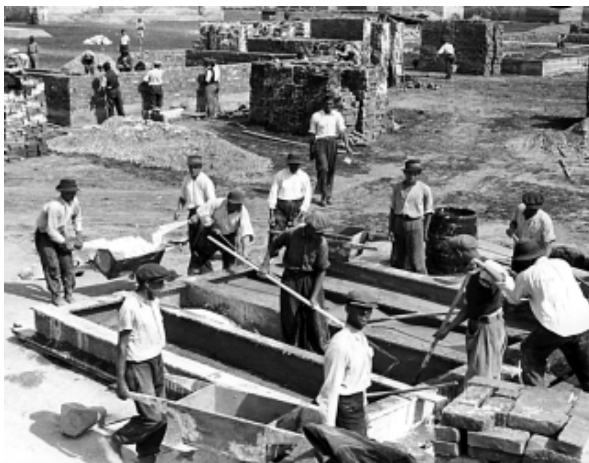
Gradnja naselja »Ante Starčević« u Donjoj Dubravi, 1941. (Arhiv Toše Dapca) Construction of the Ante Starčević housing estate in Donja Dubrava, 1941 (Toša Dabac's archive)
